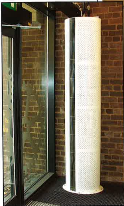
Biddle Air Systems's Invisidor STYLE, and Dimplex air curtains at Somerfield.
